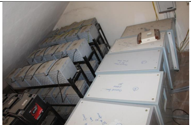
(5*5) 25K UPS Units
