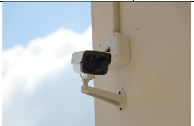
CCTV Camera (Outdoor)
