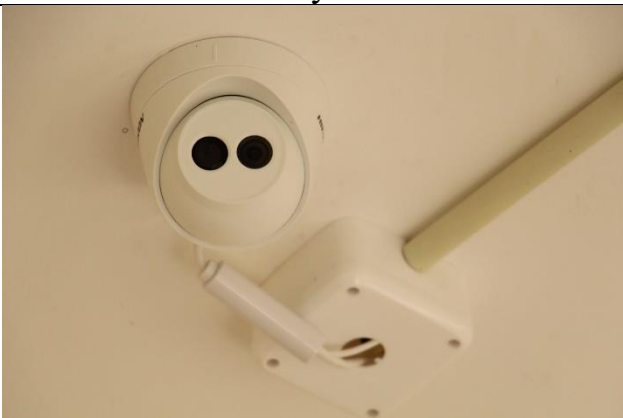
CCTV Camera (Indoor)
